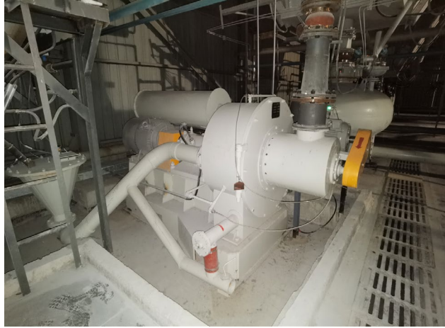
Fly ash milling facility
