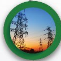
Transmission and Distribution Infrastructure
