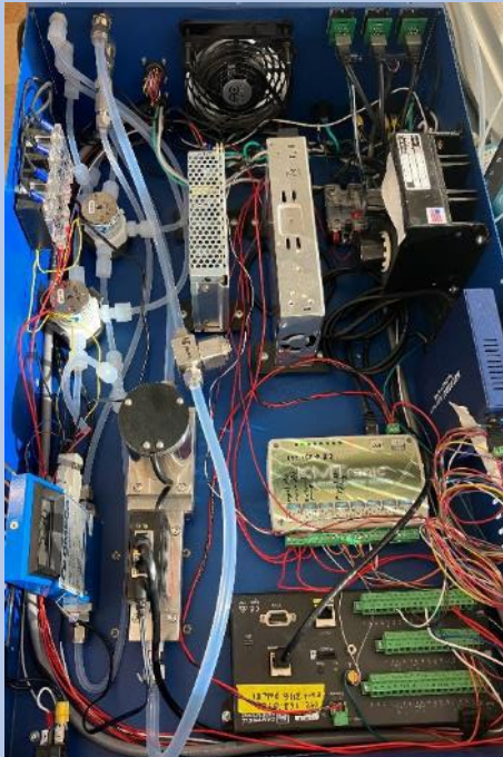
Control box CR1000x datalogger, power supplies, switching valves, communications, and flow controllers.
